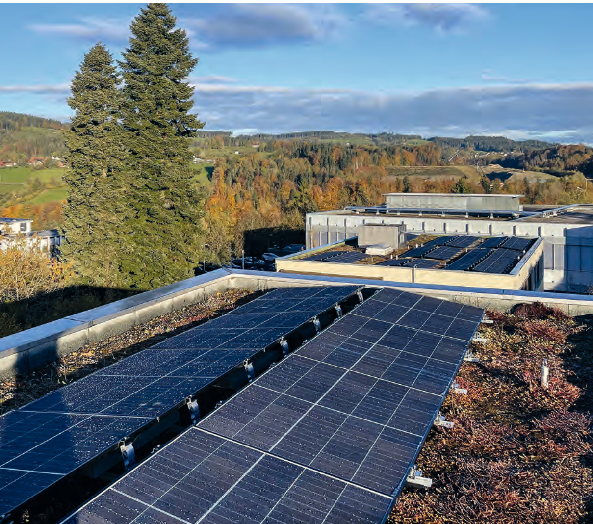
SÖMMERLI 1 MFH-Installation PV.
